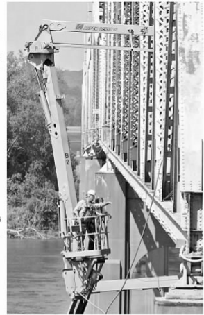
MODOT workers inspect and repair the underside of the Washington, Mo., bridge over the Missouri River last month. J.B. Forber/Post-Dispatch
